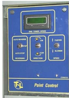
Point Control Panel
